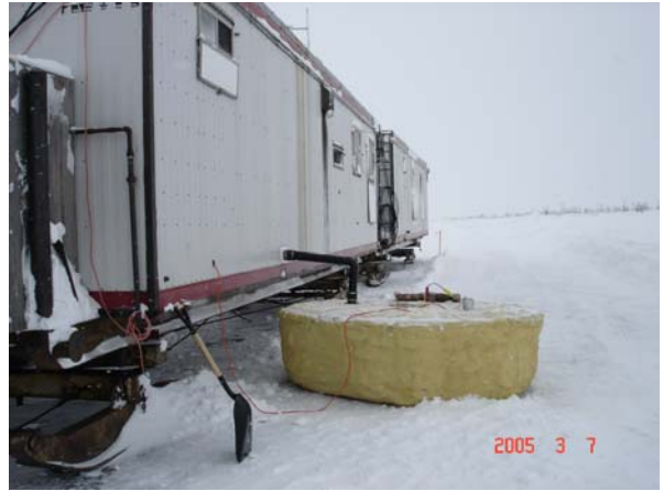
Figure 2. Waste Disposal. Sewage tank at KP-T0 TPFSA.
