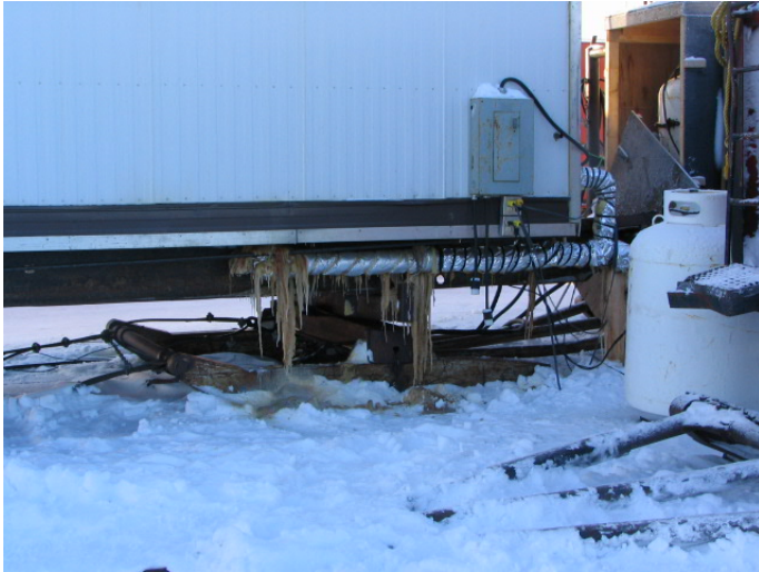
Figure 1. Sewage leaking from conveyance lines at the Grubens Sleigh Camp.
